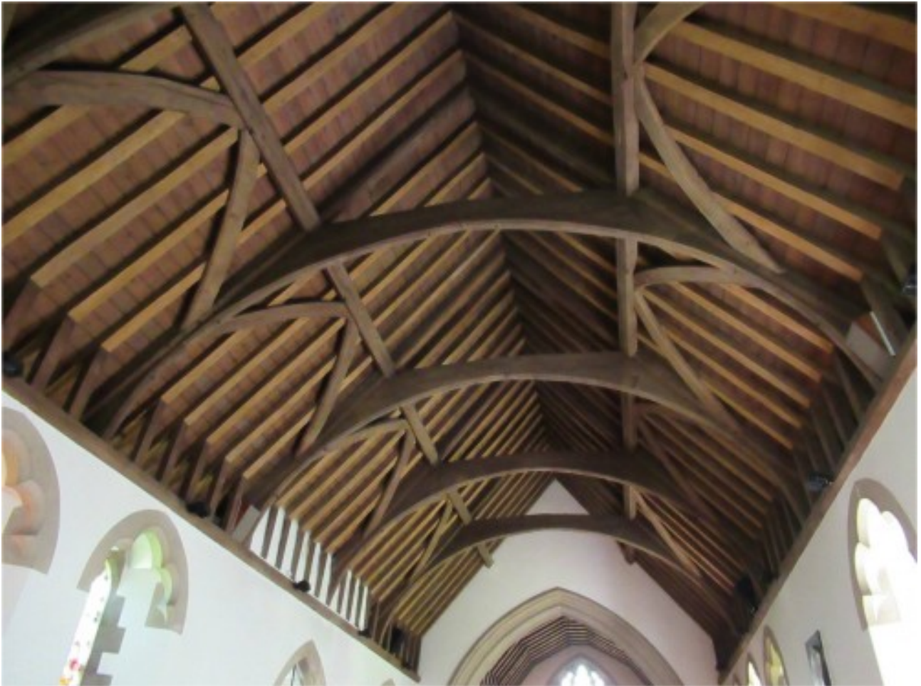
Figure 7 - View of the nave roof at Holy Trinity church. The arch brace trusses, purlins and wind braces are medieval, common rafters and boarding are Victorian. ( select picture to enlarge )
