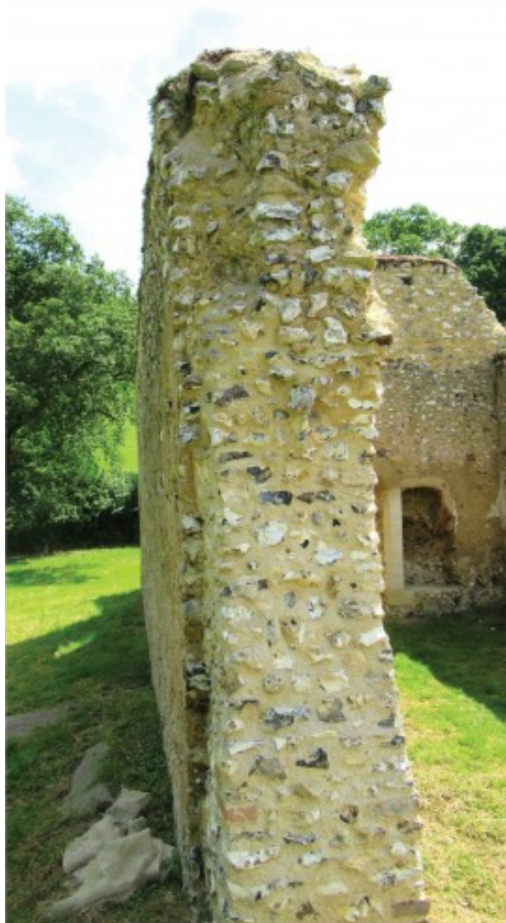
Figure 3 - The collapsed wall at St James, Bix Brand, showing solid flint construction ( select picture to enlarge )
